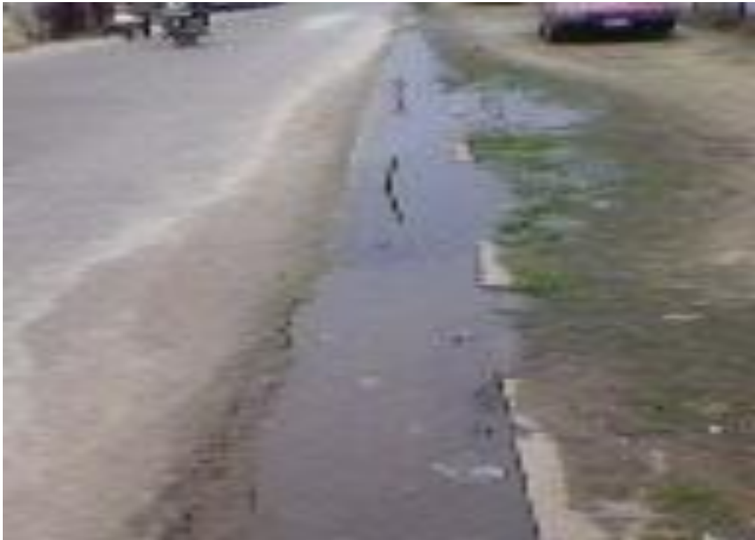
Fig. 1 Non flowing Drain in Fanikayode Road, Warri, Delta State.
