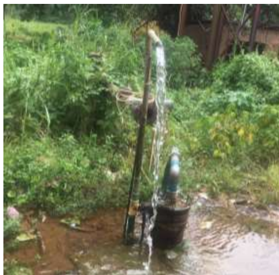
Fig. 2 Artesian well in Location A
